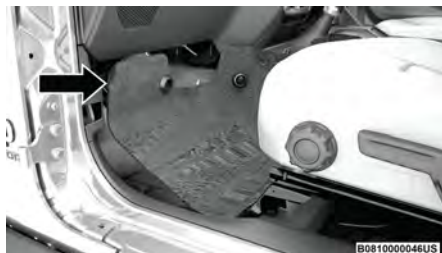
Front Carpet Pulled Away
